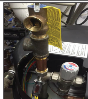
Figure 5 - Assembly Installed on Water Heater
