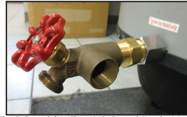
Figure 2 - Installed Combination Inlet and Drain Valve
